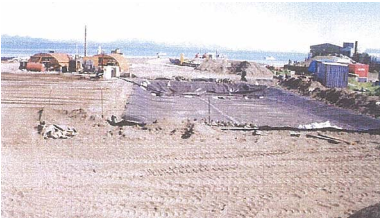
The photo above shows two soil storage pads in the foreground. One pad is complete, while the other liner awaits fill material. Each pad has a sump to collect and treat leachate. Thermal treatment units are located in the background of the photo.
