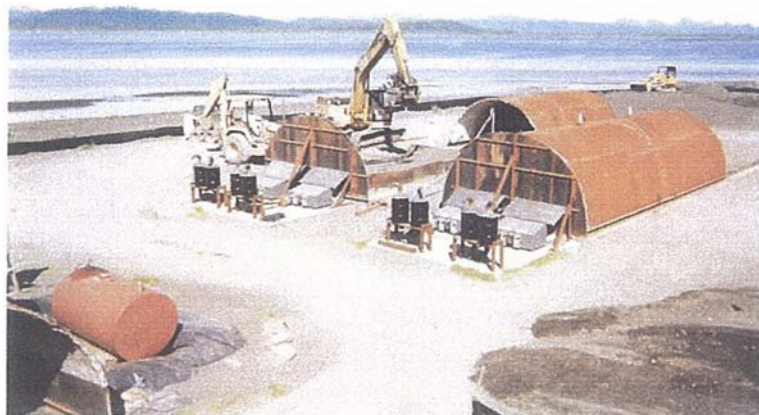
This photo shows two soil oven units. The unit in the foreground is in operation, while the unit in the background is being unloaded. No emissions have been an issue during active treatment.
